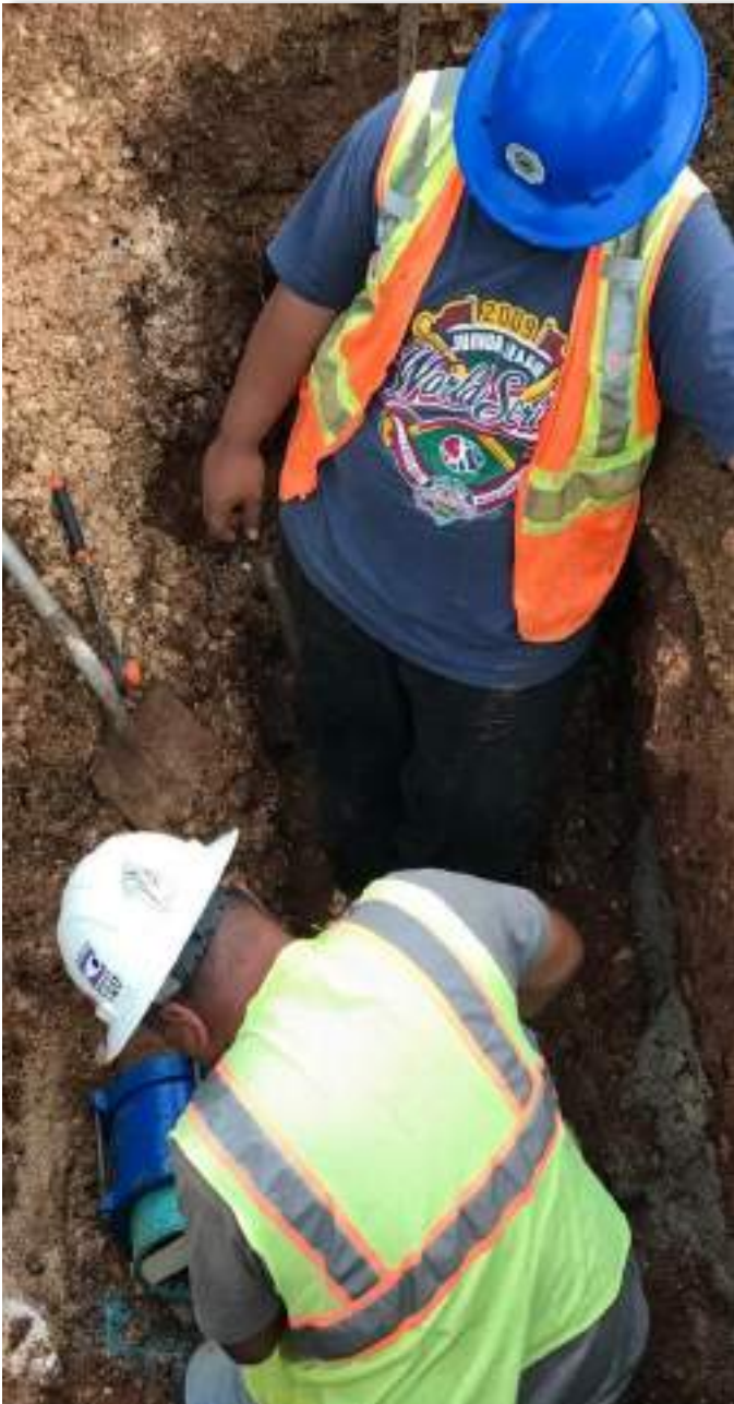
Jose Rubuenog and Oscar Stefano work to repair a leak on a six inch main water line on Airport Road.
