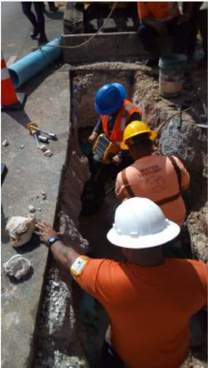
Peter Taitano, CUC Rota (bottom), Ralph Ascano, CUC Saipan (middle), and Mike Benavente, Guam Waterworks Authority (top) work together to remove rocks under an 8-inch waterline. CUC thanks the many operators from our neighbor islands of Rota and Guam who helped CUC Saipan and Tinian restore water services after Super Typhoon Yutu.
